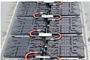
Battery charge/discharge test
